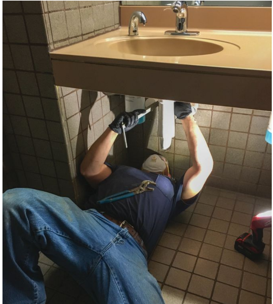
The mechanisms that make touchless faucets and soap dispensers function are hidden beneath counters. Image courtesy of Integrated Facility Services
